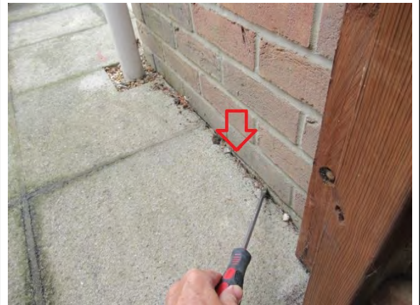
Level of damp proof course on the right side adjacent to the porch
