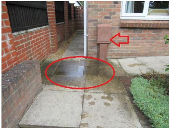
Wet path adjacent to water meter housing
